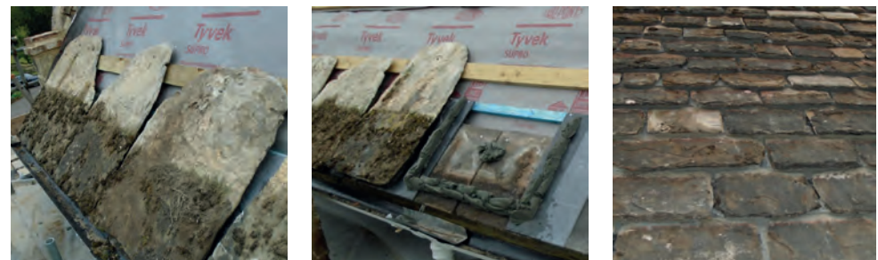
Laying of Horsham Stone slate roof with shadow slates and inconspicuous mortar
